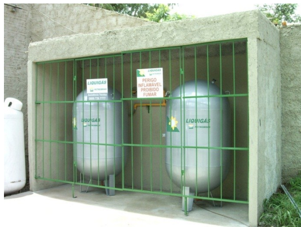
Figura 23 – Central de glp.
